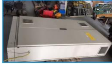
Complete Control Cabinet
