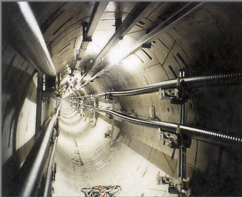
Stromtunnel in Berlin DN 3000 (6 x 380 kV)
